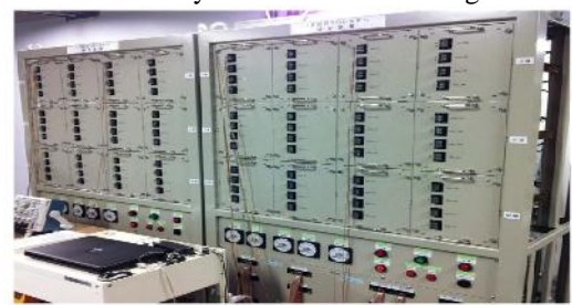
Fig.4. Photo of the three-phase 200-V, 10-kW, 50-Hz BTB system used for experiment.
