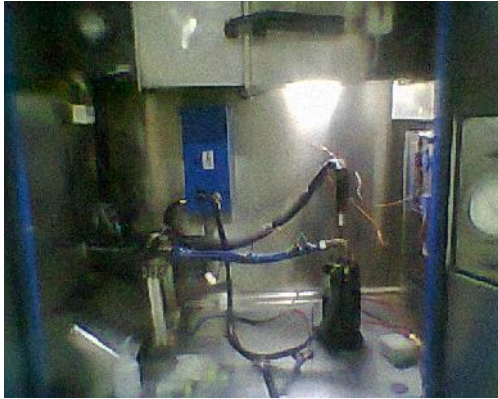
Figure 8: Compressor test cabin
